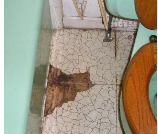
Bathroom floor damage
